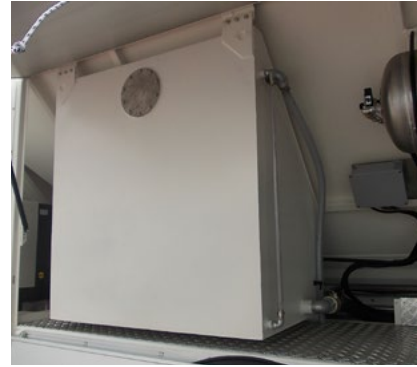
Additional water tank
